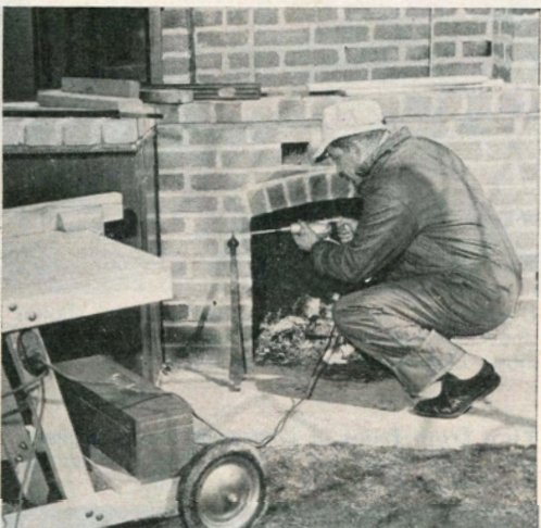
Triple outlet on leg of jointercart saves trouble of disconnecting and connecting main extension cord when drill is used.
